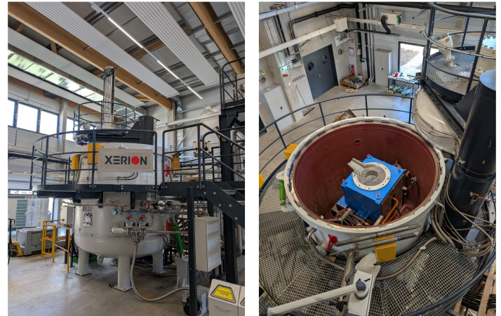
Figure 2: Pilot plant for methane pyrolysis in metallic melts in the Research Center for Hydrogen and Carbon
